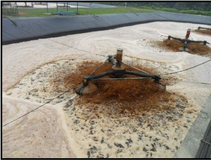
Leachate Treatment Plant
