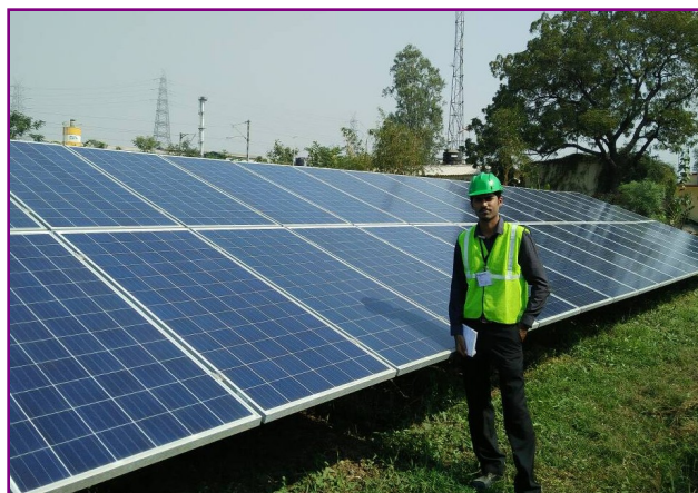
Mr Sathis with the solar harvesting system at one of JK Lakshmi Cement Factory in Kalol, Gujarat, India
