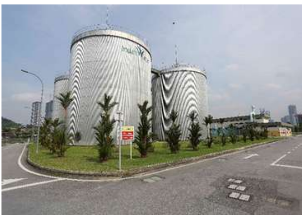
Figure 5: Biogas System at Regional Sewage Treatment Plant (Pantai 2 RSTP)
