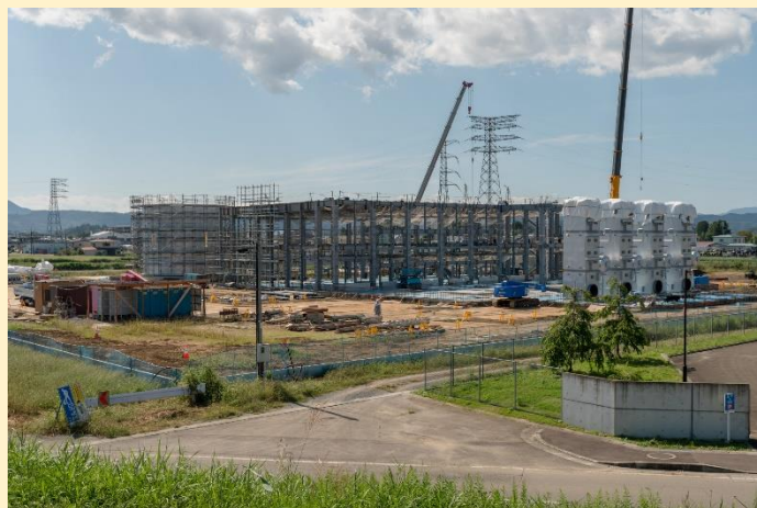
The HIS power plant in Kakuda, Miyagi prefecture, being built in 2019. The plant is now operational but HIS announced late last year that it would be selling it, citing difficulties procuring palm oil, according to Roger Smith of Mighty Earth. (Image: Mighty Earth)
