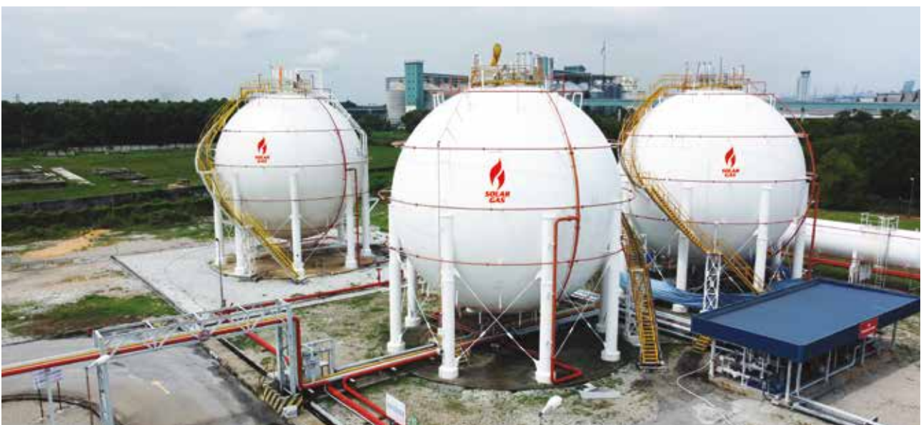
The LPG division’s storage tanks including the third tank completed in FY2022 in Westport.
