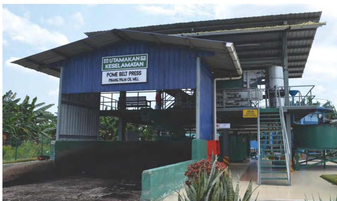
Filter belt-press which processes POME resulting in reduced formation of methane gas
