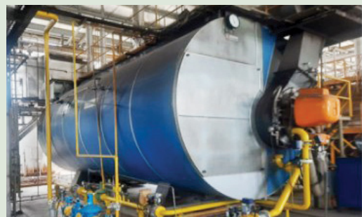
Medium Pressure Boiler 1
