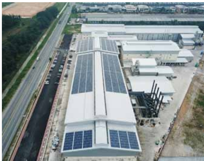
Installation of solar panels in Plant 19 focusing on sustainable, clean and renewable energy.
