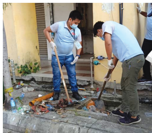
Collaboration with local authorities to clear clogged drainage in a nearby community
