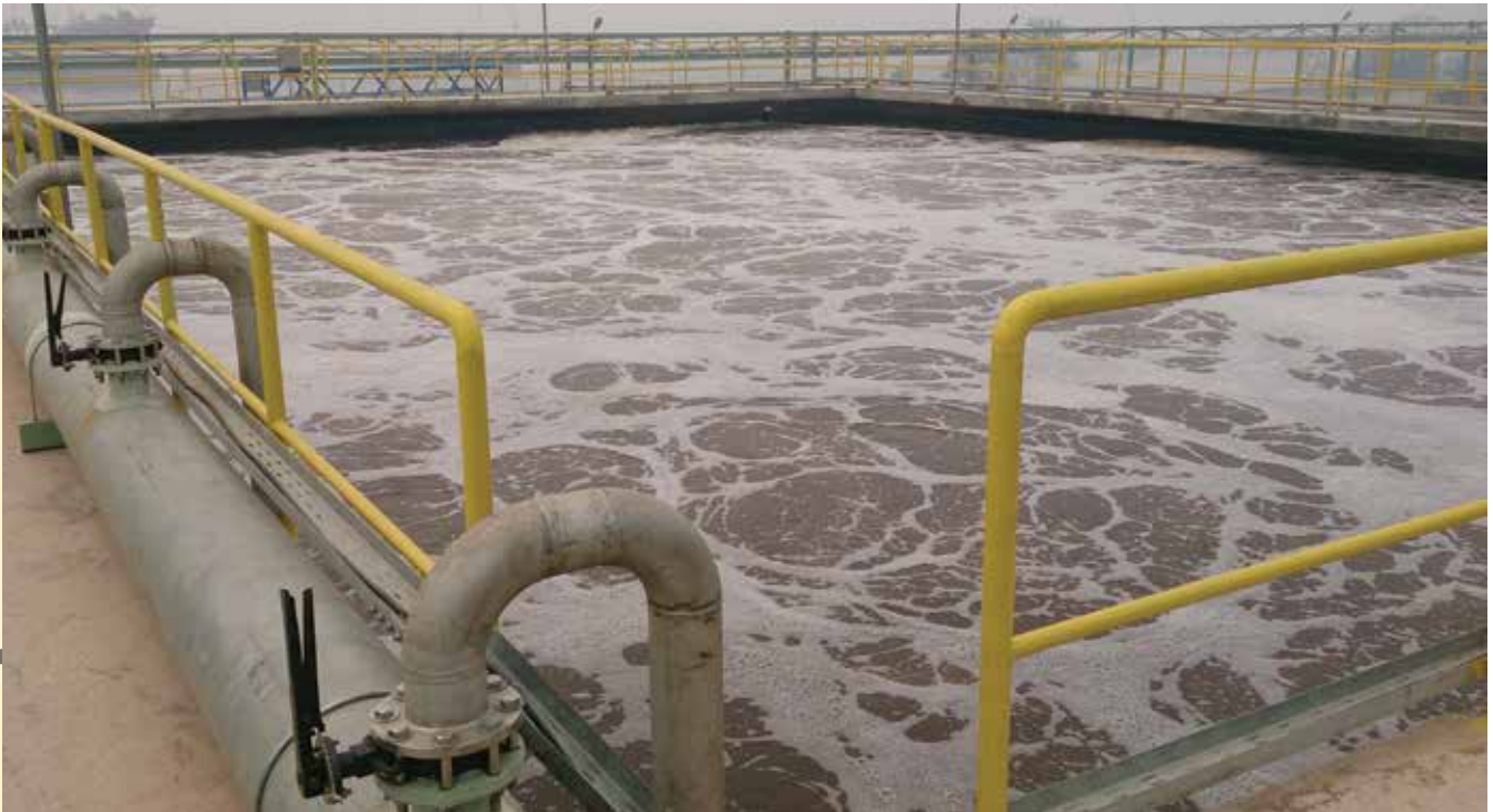
A successful Activated Sludge Process (ASP) in operation in an oleochemical, refinery, biodiesel complex in Indonesia.
