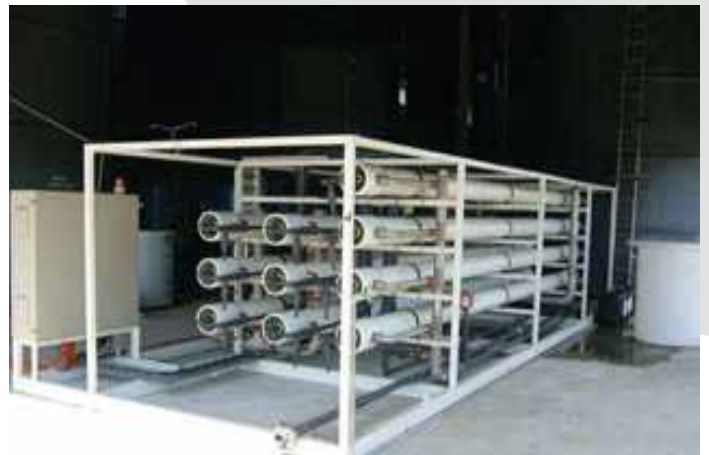
RO Installation at a large Korean Steel Plant.
