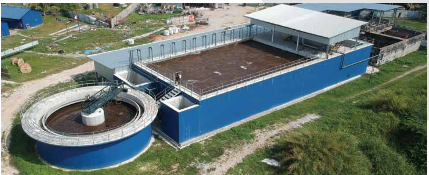
2000 m3 / day chicken processing plant in Malaysia
