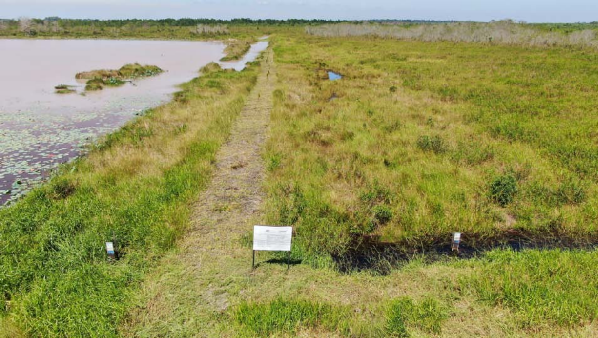
The 300m clay dyke in RMFR completed just over a three month period.
