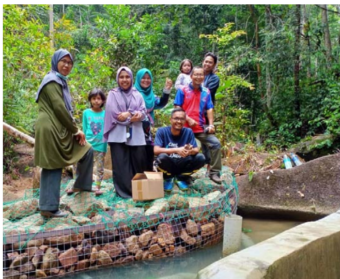
Faculty of Civil Engineering, Universiti Teknologi MARA installed a water filter cage at the source of water intake, enabling almost 500 OA community members in Kampung Kudong, Bekok, Johor to gain access to clean water. The communities were also empowered on water quality monitoring and water filter cage maintenance.
