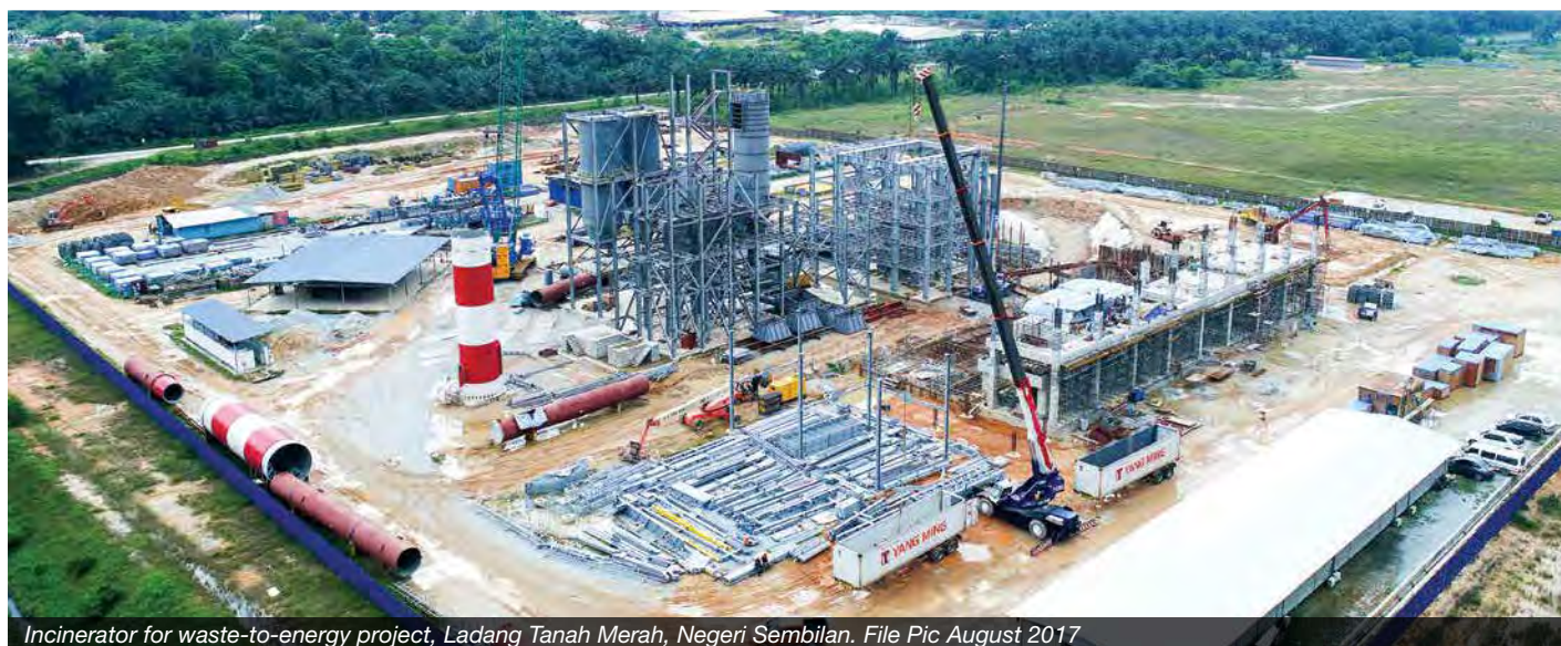
Incinerator for waste-to-energy project, Ladang Tanah Merah, Negeri Sembilan. File Pic August 2017
