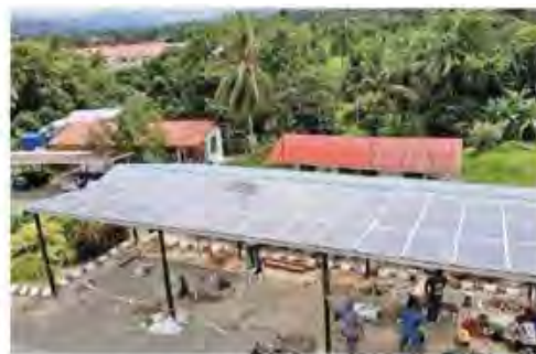
The solar power panels installed at SRJK(C) Kota Belud.
