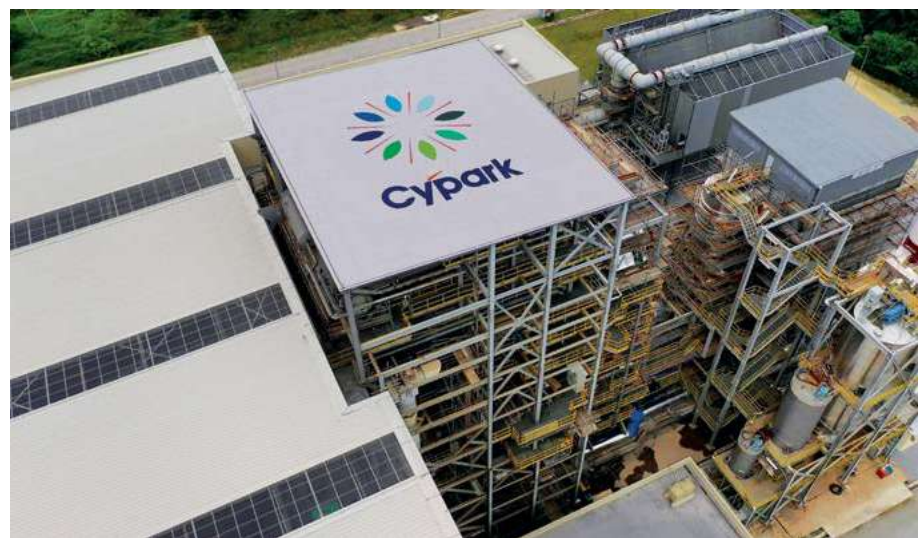
Boiler Island of SMART WTE Plant in Ladang Tanah Merah, Negeri Sembilan
