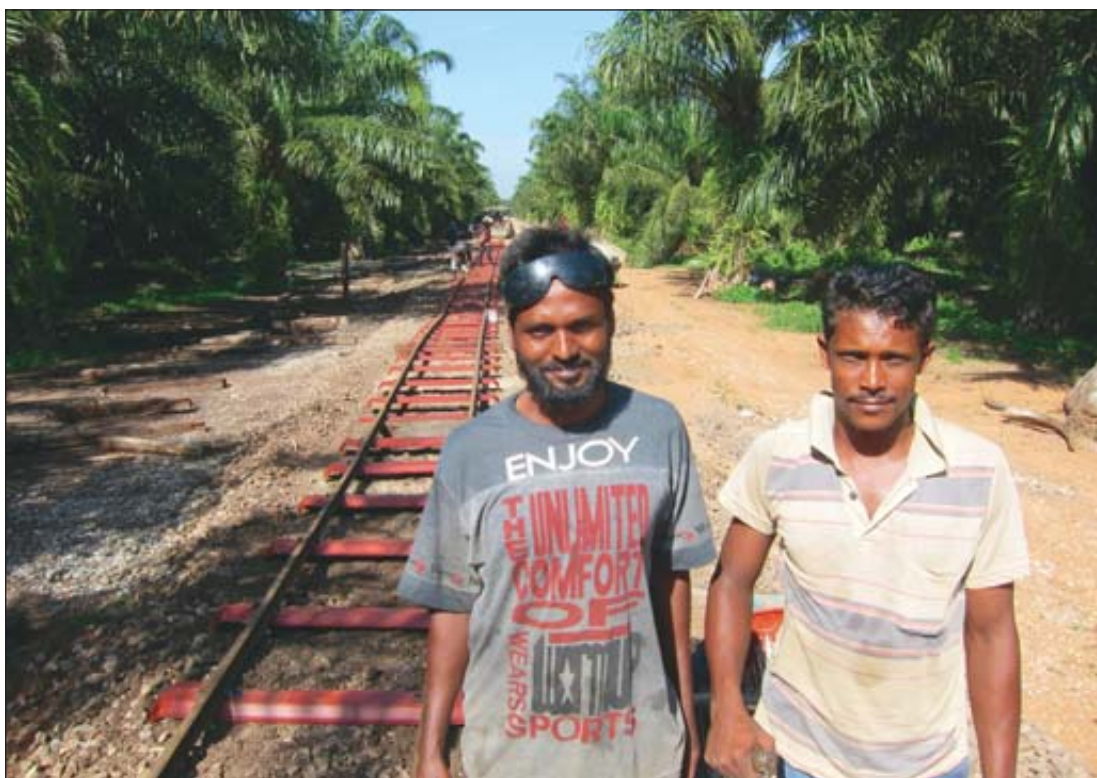
Railway gang laying steel sleepers replacing old timber sleepers. The rail system has been long established at our estates in Malaysia which has proven to be highly effective in terms of cost and quality.
