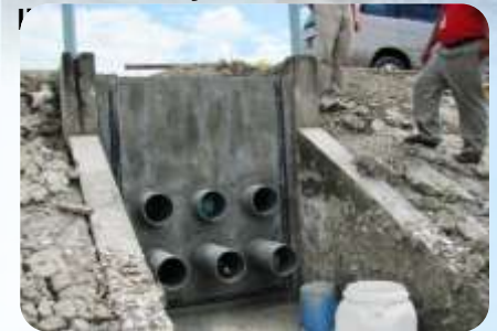
Pond outlet gate
