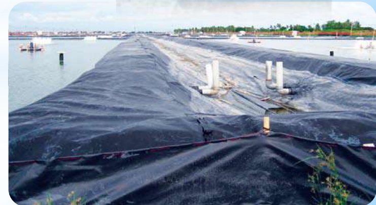
HDPE Lined secondary supply canal
