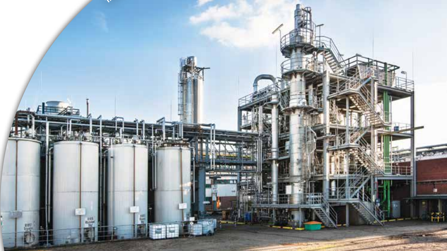
Triacetin plant at KLK Emmerich (Dusseldorf site), Germany
