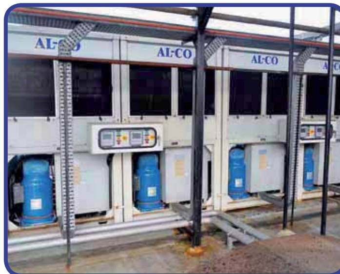
Figure: Hybrid Chiller System installed in Sri Kota
