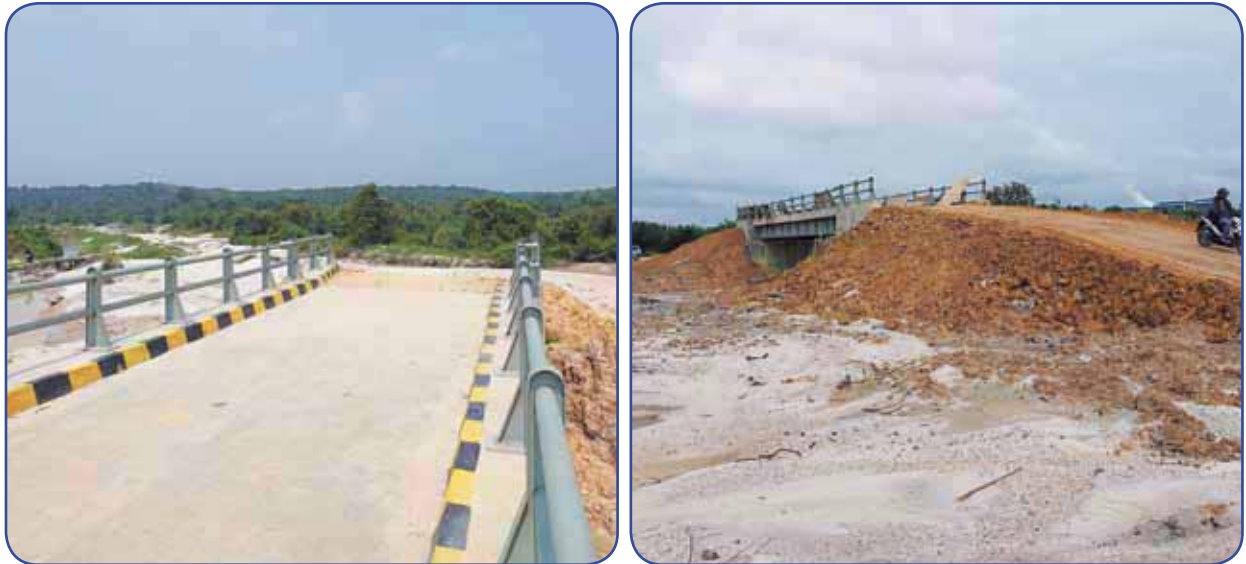
Figure: Construction of a new concrete bridge for public use at PTWan's vicinity.
