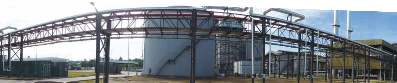
Water Tank with package boiler building
