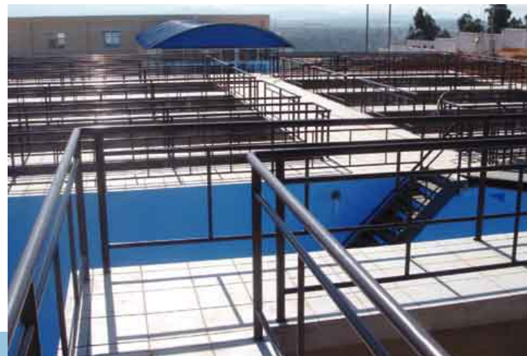
Chenggong Water Treatment Plant, Yunnan Province, People's Republic of China
