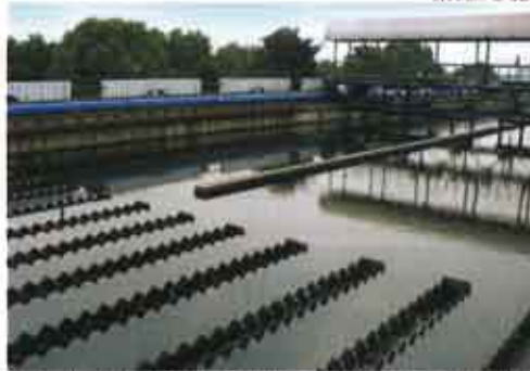
The 60mld water treatment plant in Haining City that was injected into the JV
