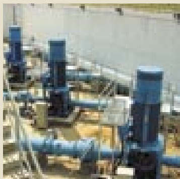
Treated Water Pumping Station at Hilir Perak
