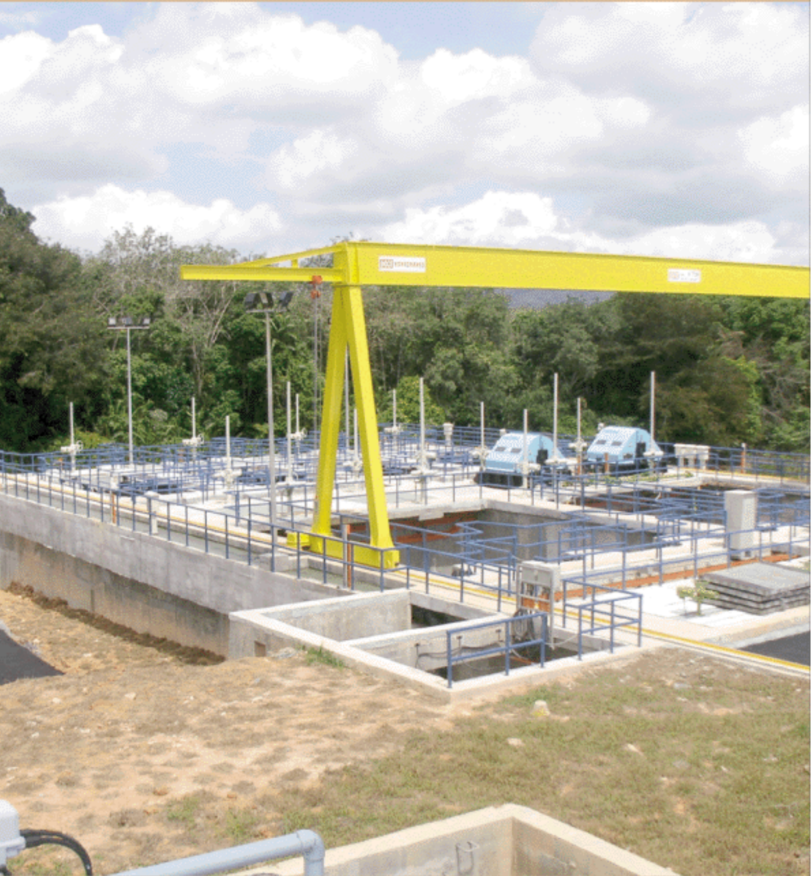
Raw Water Extraction and Treated Water Pumping Station at Kota Tinggi, Johor
