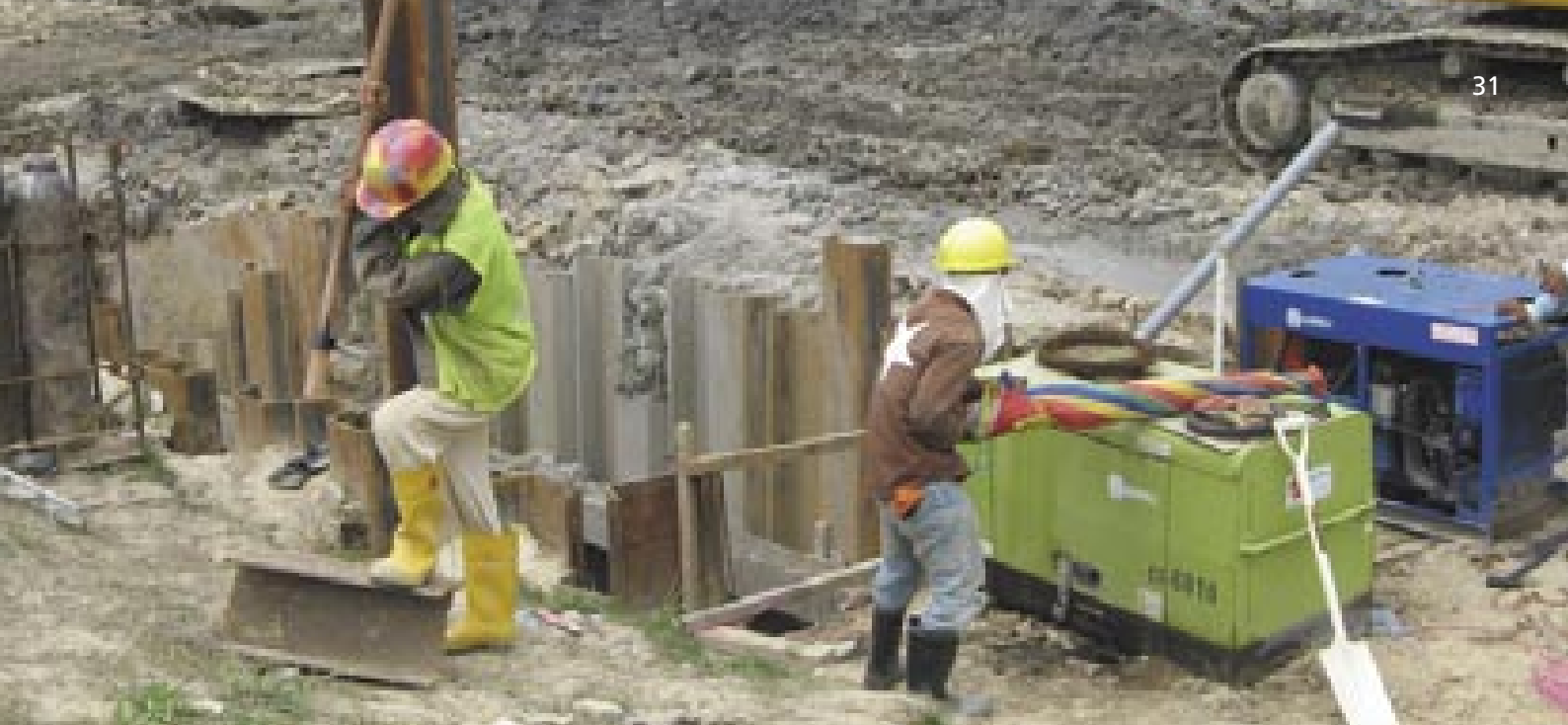
Excavation work at Jalan Pintas to lay pipelines for the Kota Kinabalu Sewage project
