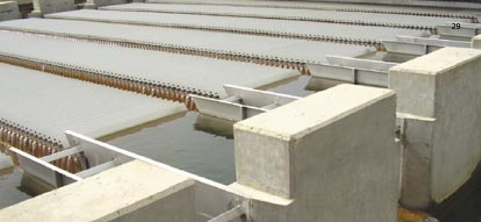
Lamella Clarifier at Lancang Water Treatment Plant, Stage 1, Melaka
