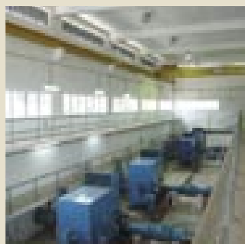
Pumping room at Kuala Jelai Water Treatment Plant, Negeri Sembilan
