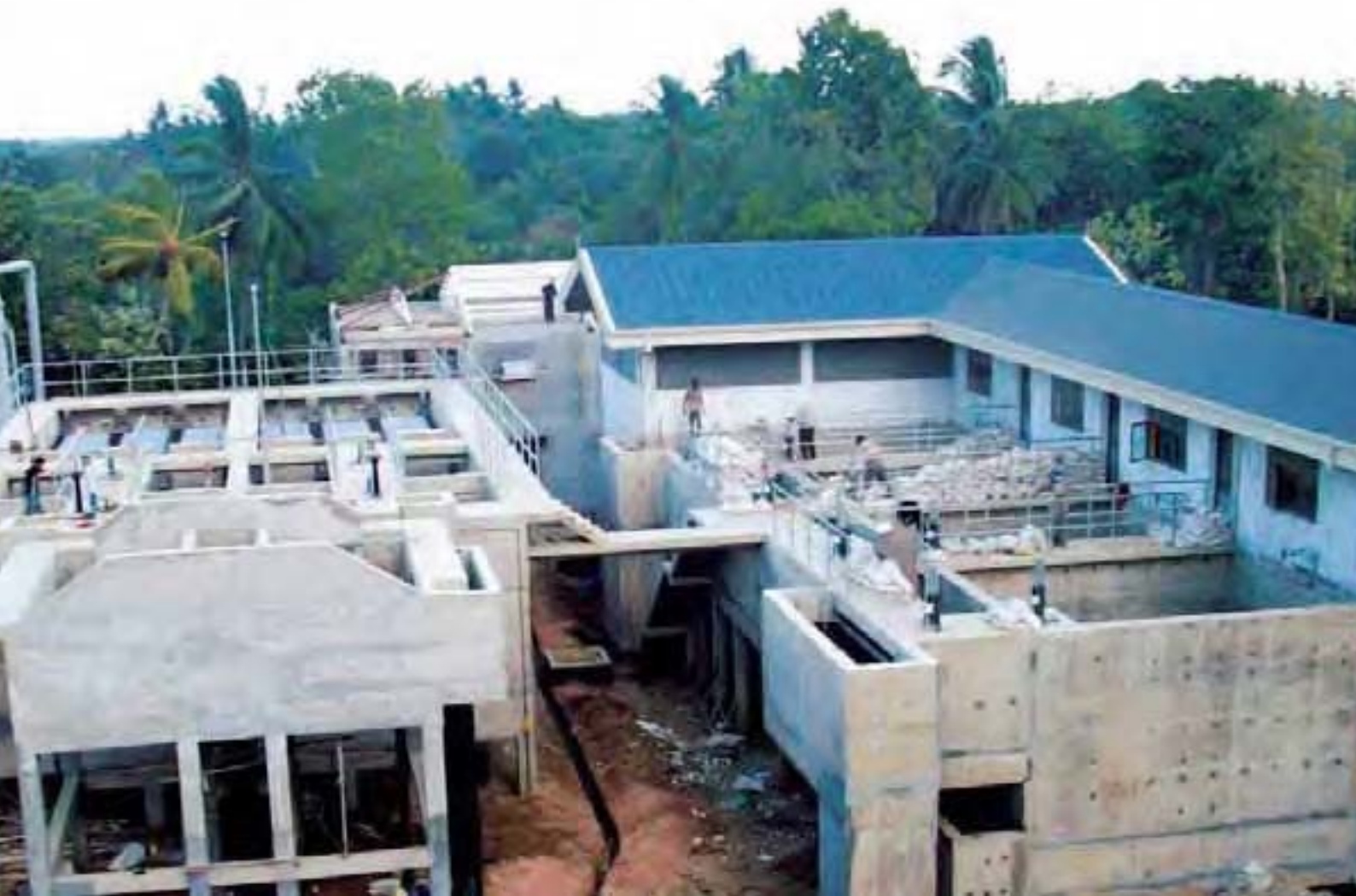
Overview of Process Plant for Hambantota Water Supply Project, Sri Lanka.
