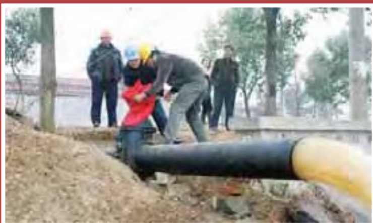
Pipelaying works for Yizheng treated water supply project, Yizheng City, Jiangsu Province, China
