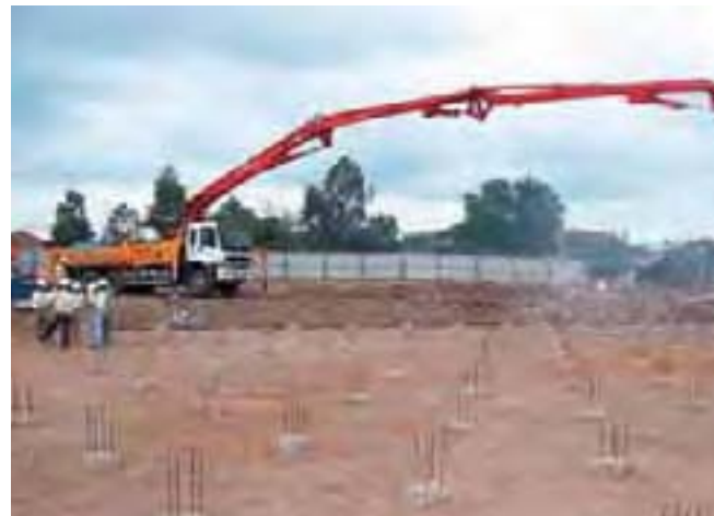
Casting lean concrete for Flocculation and Sedimentation tank for Nhon Trach Water Supply Project, Vietnam
