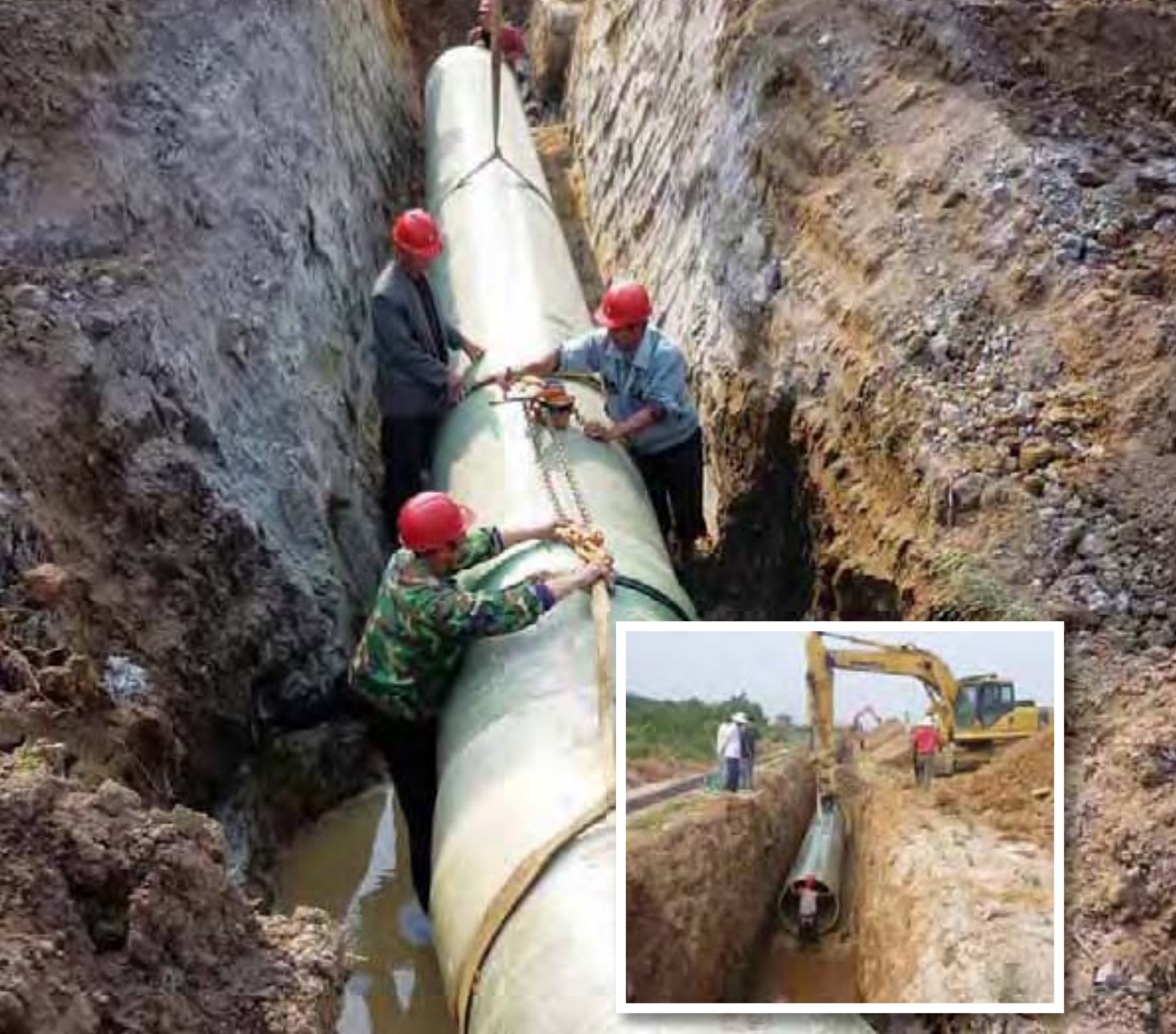
On going pipe laying works for Nan An Raw Water Supply Project, Nan An City, Fujian Province, China
