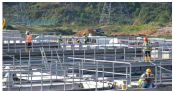
On-going construction of Clarifier & Chemical Mixing Chamber at Langat 2 Water Treatment Plant
