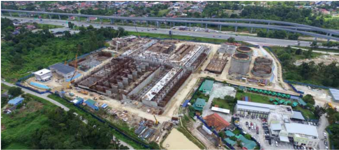
Langat Centralized Sewage Treatment Plant will accommodate an inflow of 920,000 P.E. upon its completion.
