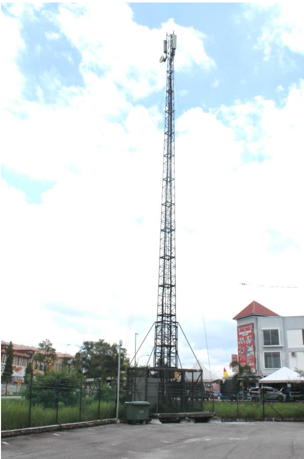
Foto 6: Portable Base Transceiver Station (BTS) - mast
